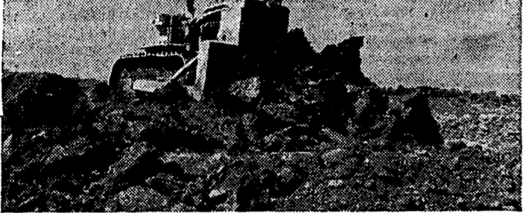
BEAR for work is this new International TD-25 crawler tractor, here moving huge load of earth on runway extension project at Chicago's jet-age O'Hare International airport.
