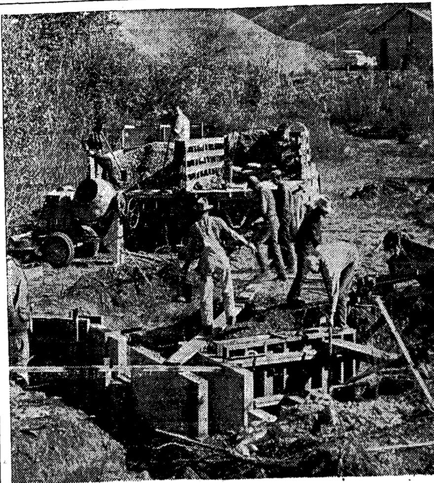
Idaho Fish and Game Department construction crew finishes pouring concrete structures for another fish screen in the Salmon River region. This unit is located on the North Fork of the Salmon River and is designed to keep young salmon from entering irrigation ditches and canals on their downstream trip to the ocean. Approximately 250 screens will be installed before the project is completed.
