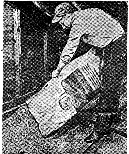
Zonolite vermiculite insulation being installed over ceiling of dairy barn at Sinnissippi Farms, Oregon, Ill.
